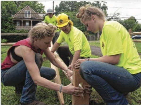
STAFF PHOTO/CAROL LOLLIS Twins Shelby, left, and Cierra Frey, 17, and Jacob Oulmette, 16, at back, part of the summer grounds crew at Smith Vocational High School, work with Mark Nevin, head of the Horticulture Department at the school, on a new fence running along the entrance to the school. Freshmen start Aug. 25 while the rest of the students return Aug. 28.
